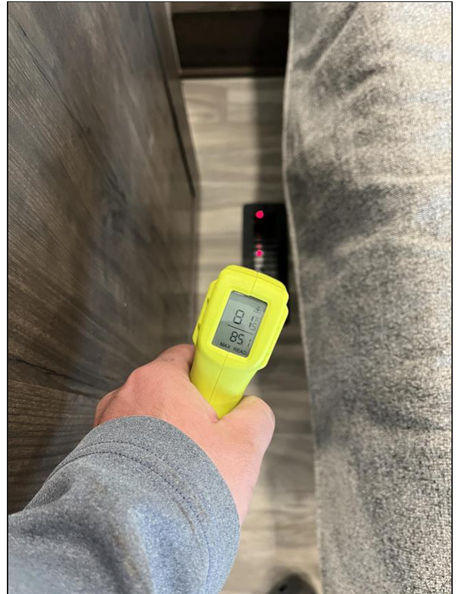
Bedroom weak air discharge
