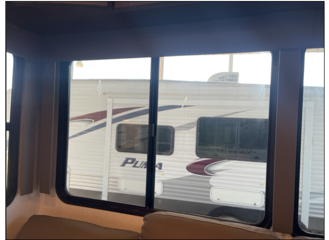
Missing window cover
