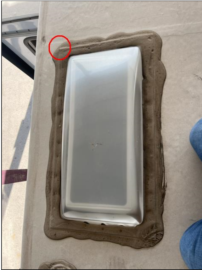
Location of Sealant Crack
