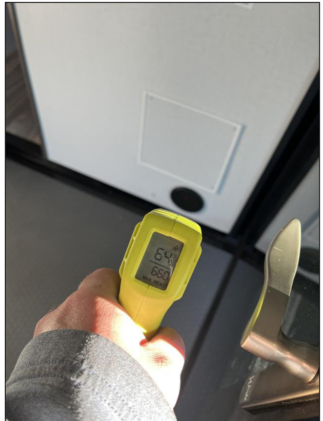
Garage no air discharge
