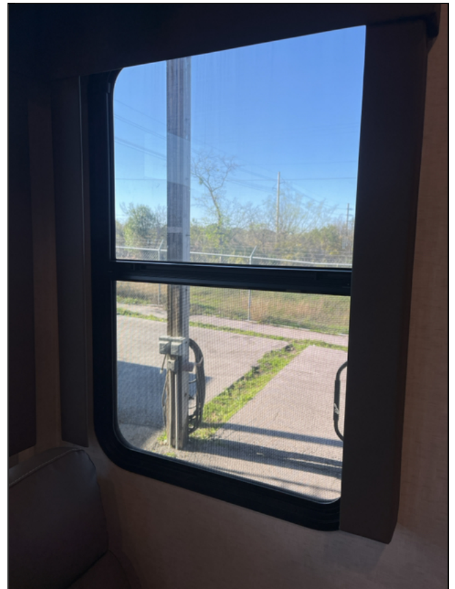
Missing Window Cover
